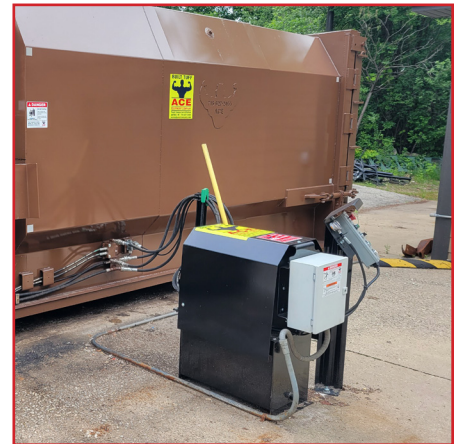
Hand-Built Power Units
